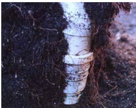
FIG. 9 MELALEUCA ROOTS SURROUNDING THE JOINT
