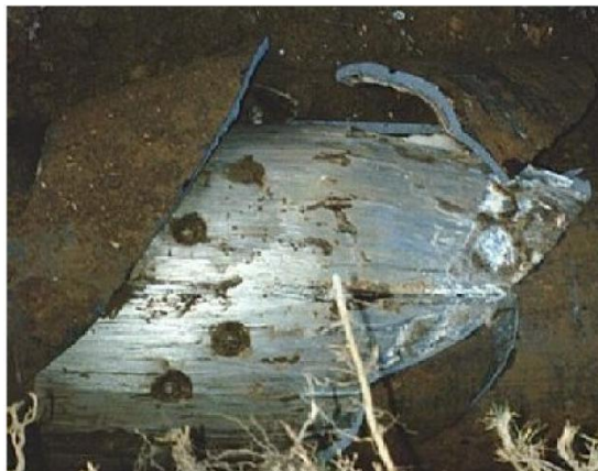
PIPE BURSTING HEAD BREAKING OPEN CAST IRON PIPE AT AN EXCAVATION - PHOTO COURTESY OF CLM TRENCHLESS
