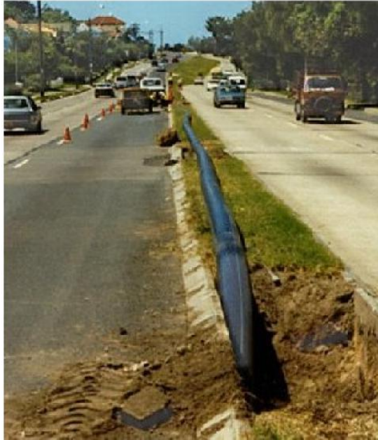
PE BEING DRAWN BEHIND PIPE BURSTER ON PITWATER RD, SYDNEY – PHOTO COURTESY OF CLM TRENCHLESS
