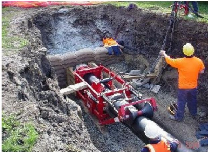
SWAGE LINING DN500 SHOWING REDUCING DIE AND ROLLERS, HOBART TASMANIA – PHOTO COURTESY CLM TRENCHLESS
