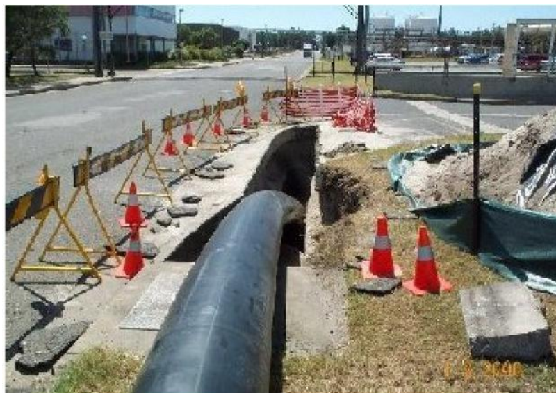
SLIP LINING WITH DN500 PE, BOTANY NSW – PHOT COURESY OF CLM TRENCHLESS
