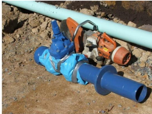
TYPICAL ASSEMBLED FLANGED VALVE WITH PUDDLE FLANGE ADAPTER. FLANGES WRAPPED TO PROTECT BOLTS
